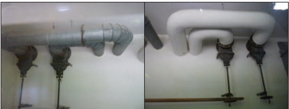
Ill. 53f.: Thick pipes in the room behind and in the area above the Dachau “gas chamber.”
