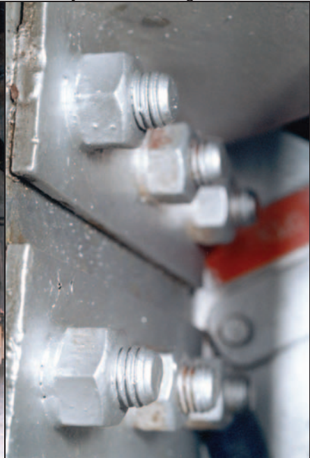
Fig. 106: Closeup of bolts on door hinges.
