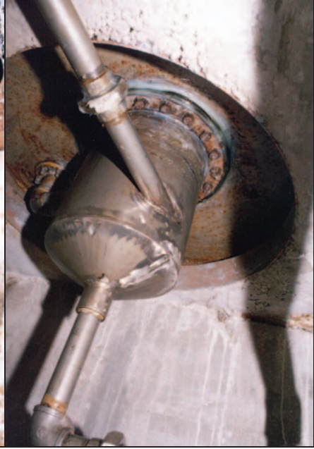
Fig. 104: View of stainless-steel plumbing and chemical container directly under seat in gas chamber.
