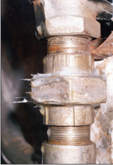
Fig. 103: Closeup of plumbing underneath the gas chamber covered in Vaseline to indicate leaks.
