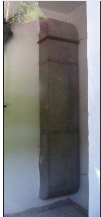
III. 56: Warm-air-supply shaft behind the Dachau gas chamber.
