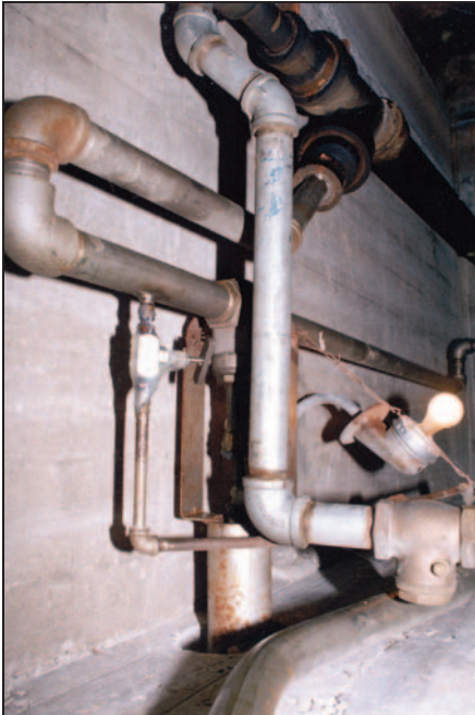
Fig. 105: Portion of plumbing and sewage system connecting chemical room to gas chamber.
