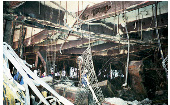
Fire damage in WTC 5 (2002 NIST survey of fires that resulted in total or partial collapse).
