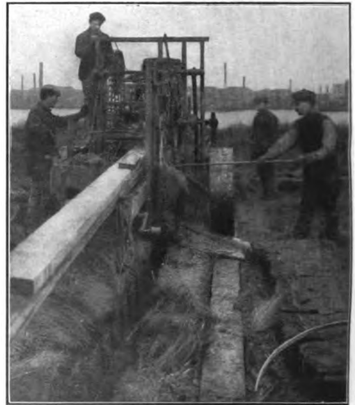
EXTERMINATING SWAMP MOSQUITOES DRAINING THE MARSHES BY MEANS OF A MACHINE THAT DIGS A MILE OF TRENCHES A DAY
