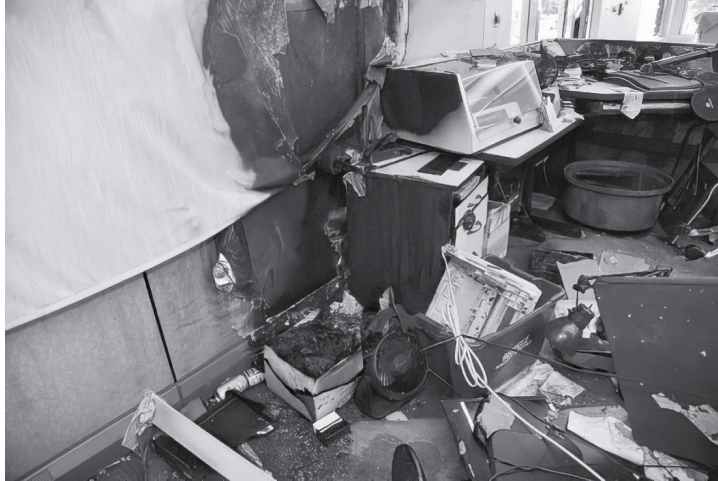
An office in the Justice Center in Portland was destroyed by rioters on May 29, 2020. Photo: U.S. Attorney's Office
