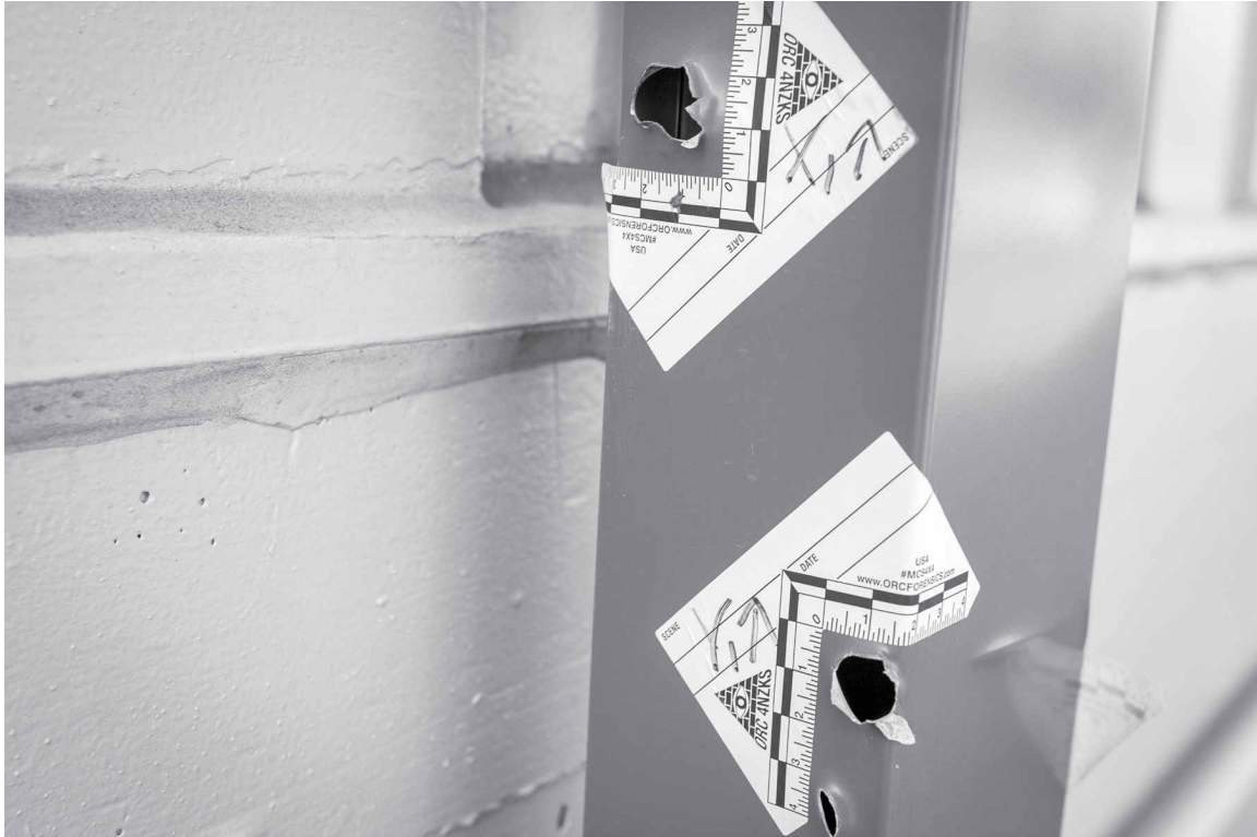
Bullet holes at the Tacoma, Washington Immigration and Customs Enforcement facility. Photo: Andy Ngo
