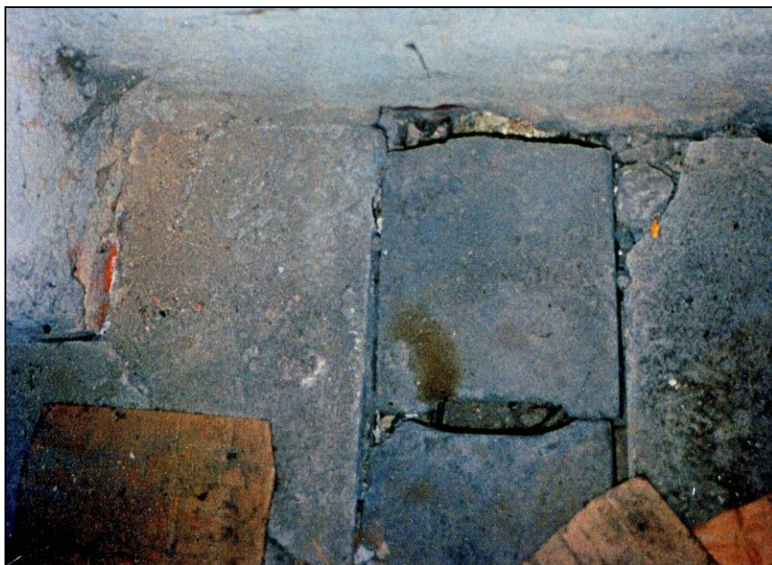
Document 16: Water run-off in floor of gas disinfestation chamber in BW 5a at Birkenau. © Carlo Mattogno.
