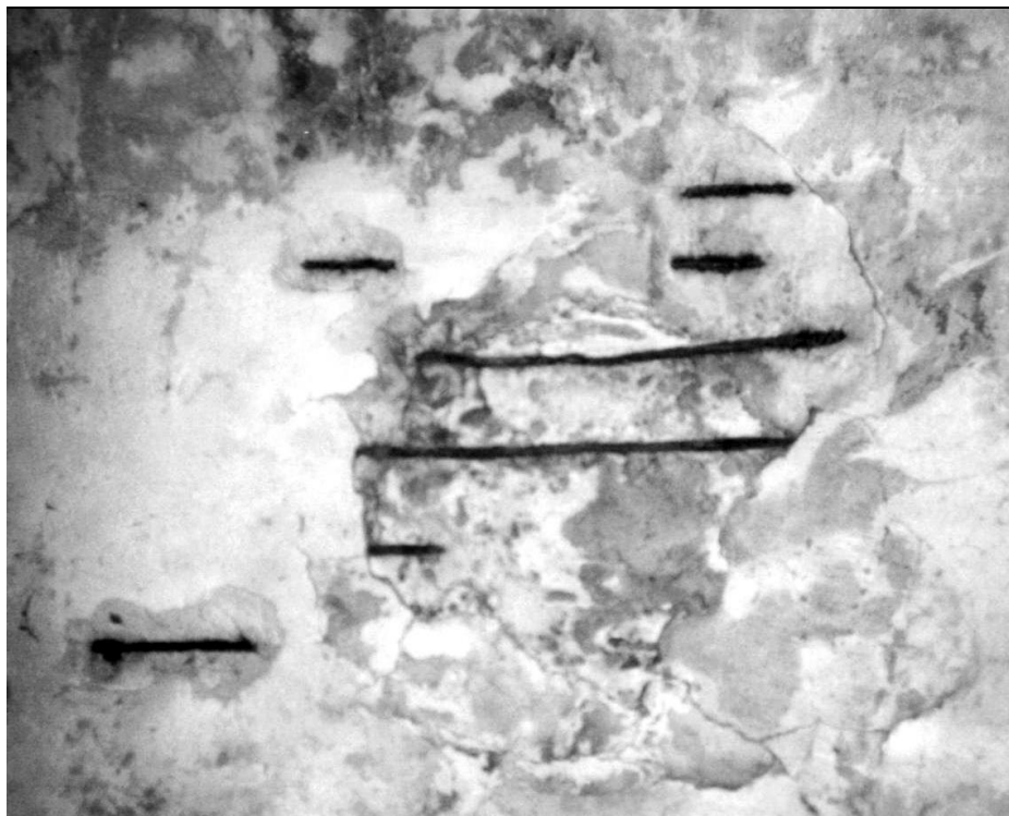
Document 22: Photo of opening no. 4 in the roof of the washing room. © Carlo Mattogno
