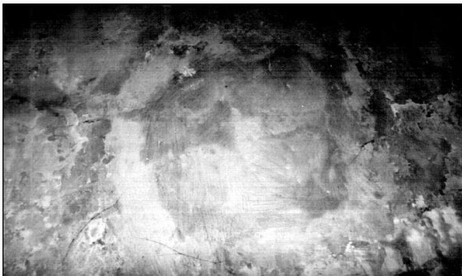
Document 20: Photo of opening no. 2 in the roof of the morgue. © Carlo Mattogno
