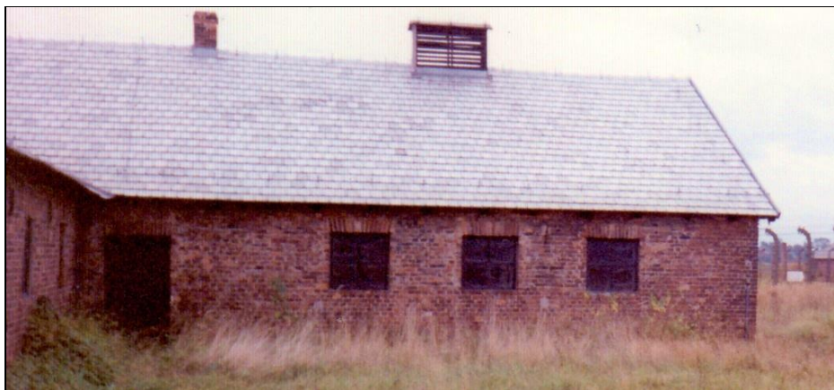
Figure 167: Disinfestation wing of Building 5a, northern wall, with little staining. (© C. Mattogno 1991)
