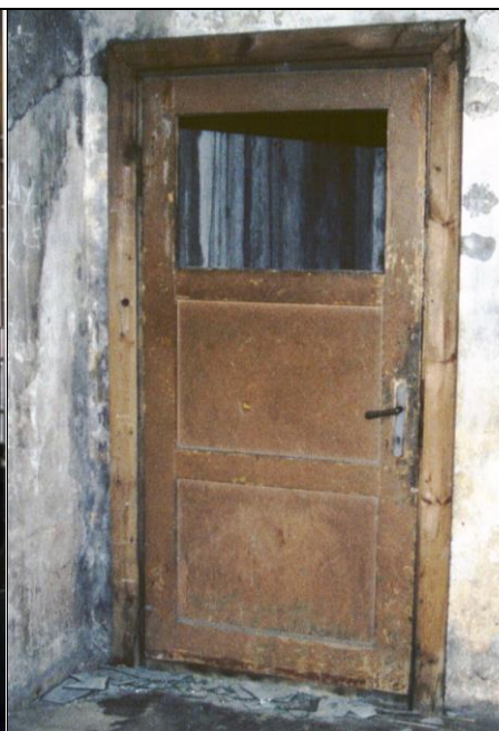
Figure 11: Door in the room of Crematorium I at Auschwitz (Main Camp) which has been presented for decades to museum visitors as a homicidal gas chamber. This unstable, leaking door with a window pane once separated the washroom from the laying-out room. It could never have served as a gas-chamber door. Such discrepancies between what Leuchter expected to find in Auschwitz and what he found induced him to write his expert report.
