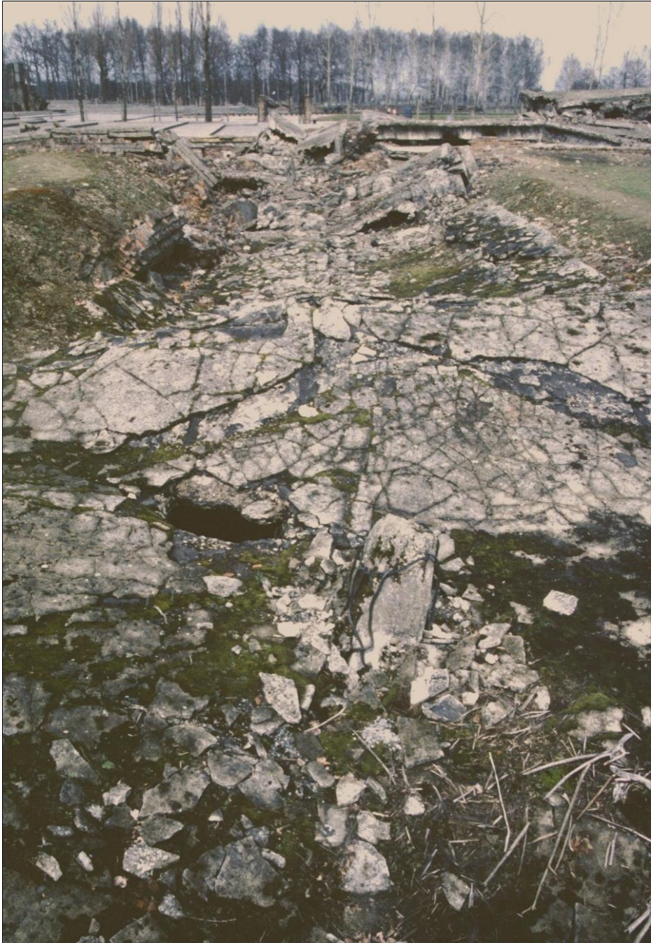
Figure 62: Morgue #1 of Crematorium II in Birkenau, collapsed roof, February 1997. Background: the collapsed crematorium building to the right, the memorial to the left. Foreground: The last of the seven concrete pillars poking through the roof. A meter or so to the left: a hole chopped through the roof to gain access to the area below (see Figure 84, p. 139). (February 1997)
