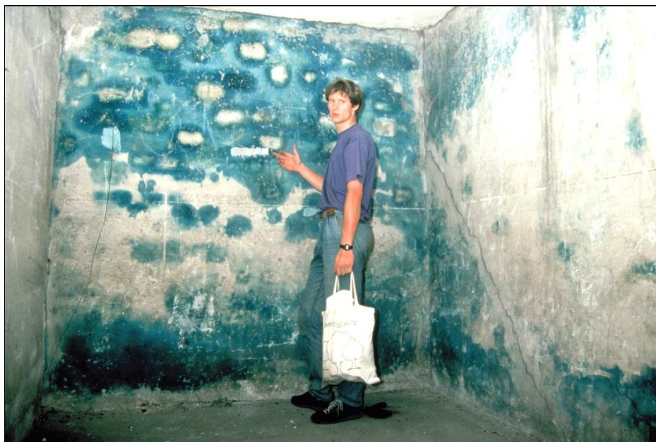
Figure 146: Room located in the northwest of the disinfestation wing of Building 5a (Room 4 in Figure 40) with the author. The exterior walls are located in the background and to the right, showing intensive blue discolorations caused by Iron Blue. Sampling locations of Samples 9 and 11 are visible. On the left in the picture is the interior wall, erected during the conversion to a hot-air-disinfestation chamber. Sample 10, with a slightly positive cyanide content, was taken from this wall.
