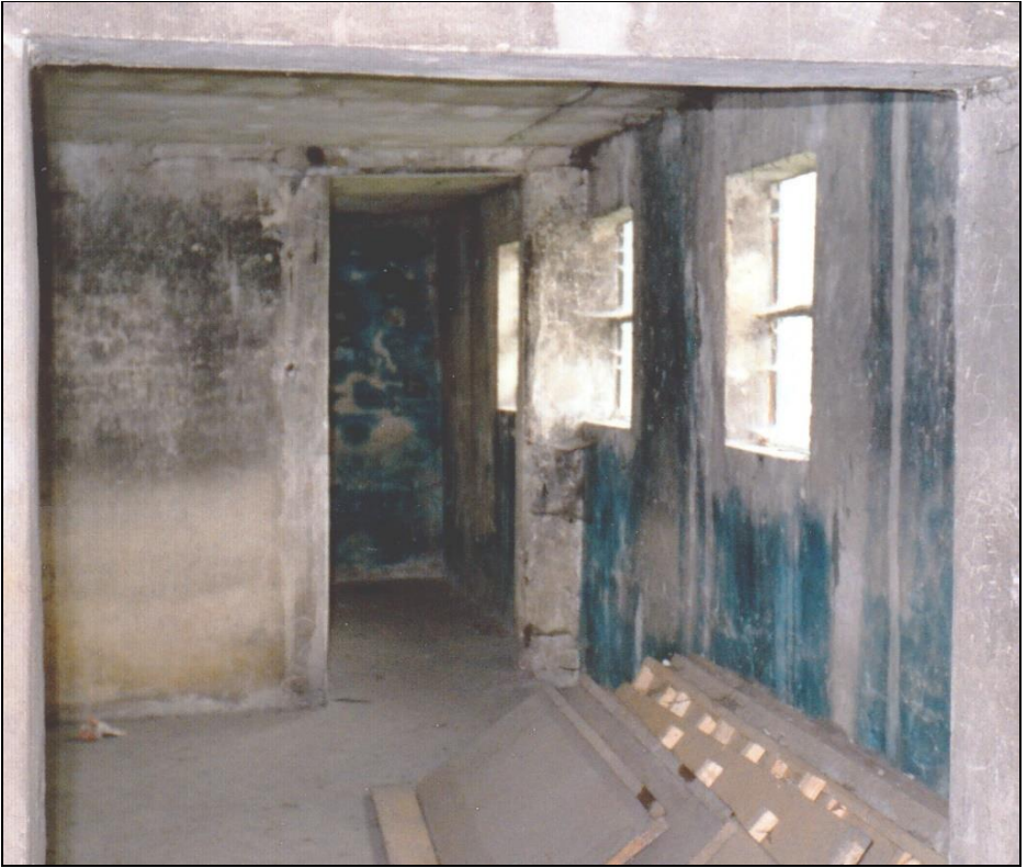
Figure 160: Disinfestation wing of Building 5a, with northern external wall to the right, with Room 5 in the foreground and Room 4 in the background (see Figure 40). (© C. Mattogno 1992)
