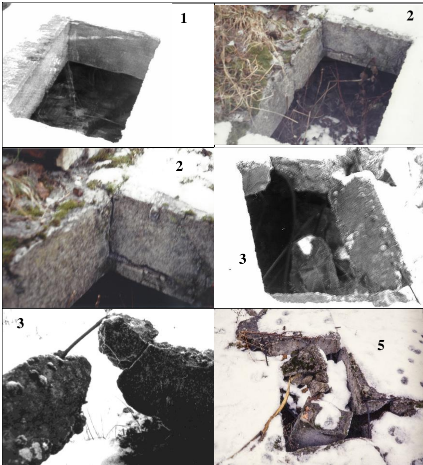
Figures 91-96: Four of the five properly constructed ventilation holes in the ceiling of the furnace room on the ground floor, Crematorium III (no. of holes indicated; #2 and #3 twice); condition: December 18, 1991. Note the cracks caused by the explosion, especially at the corners. The close-up photo of Hole #3 (third row on the left) shows a reinforcement bar running around the hole and still holding the concrete fragments together.
