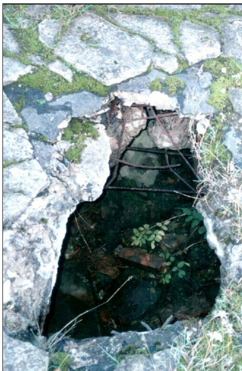
Figure 84: Hole in the ceiling of Morgue #1 ("gas chamber") of Crematorium II, entry to the still-accessible part of the morgue. Maximum width: 50 cm; maximum length: 86 cm. © 1992 Carlo Mattogno
