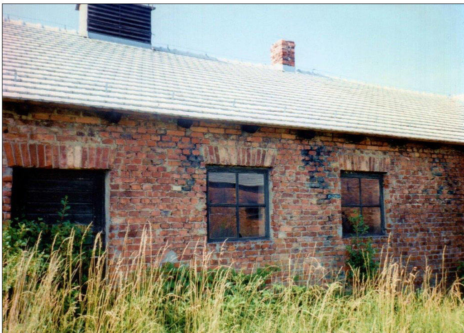
Figure 161: Disinfestation wing of Building 5a, southern wall (of Rooms 4 and 5 in Figure 40). (© C. Mattogno 1992)
